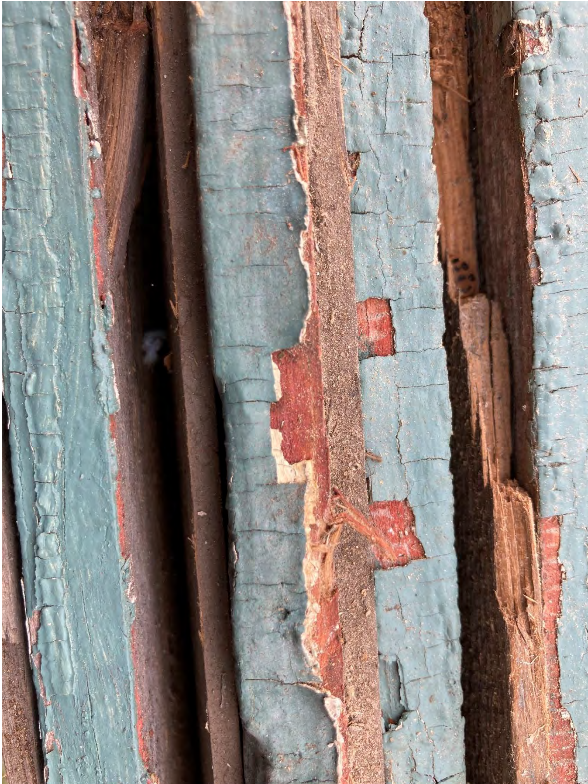
Figure 11 – Detail of siding showing color layers.
