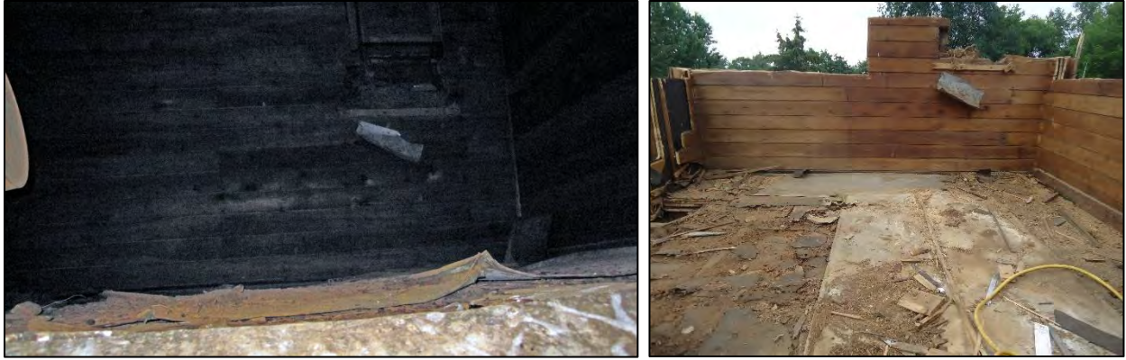
Sheets of galvanized metal with standing seams covered the tank room floor. These photographs were taken from the tank room doorway facing north before (left) and during (right) disassembly. (Photographs by Paul Bergson, left, and Curt Richter, right)
