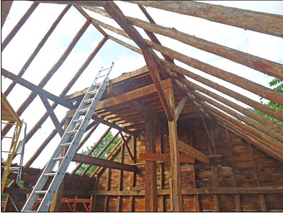
Left: The structure supporting the tank room was visible when the barn was disassembled. (Curt Richter photograph)
