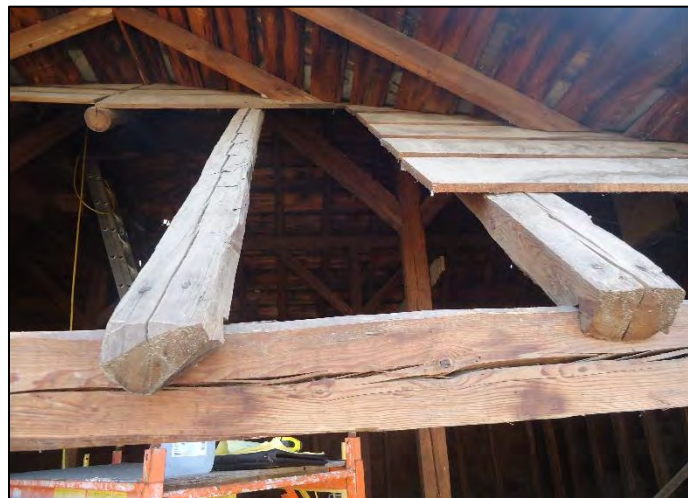
Where the east and west sections intersect, the rafter tails of the east roof were on the interior. They were trimmed differently than the rafter tails exposed on the exterior. (Curt Richter, photographer)
