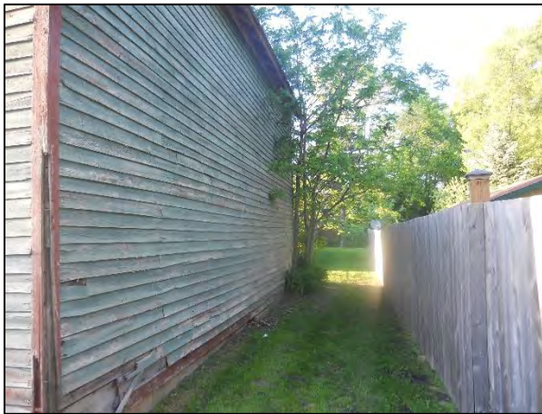
Filled-in openings on the east wall before (top) and after (center) the interior sheathing was removed. The exterior clapboard (bottom) showed no evidence of the openings. (Photographs from Two Pines, top; Curt Richter, center and bottom)
